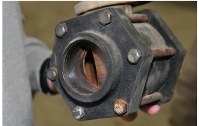
Open valves to allow water that is trapped behind the ball to flow out.
