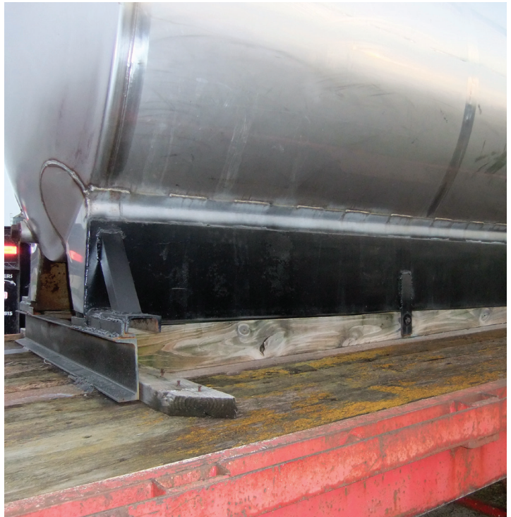
This is a good installation of a stainless tank on a trailer. Notice that the tank slopes down, which allows the operator to completely empty its contents and clean it easily. It is also mounted securely to the trailer with steel and wood bracing.
