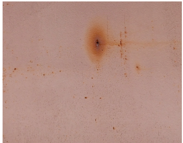
This mild steel tank has pinholes in it that are so small, the fertilizer just weeps out of it. Mild steel is susceptible to damage from corrosive materials.
