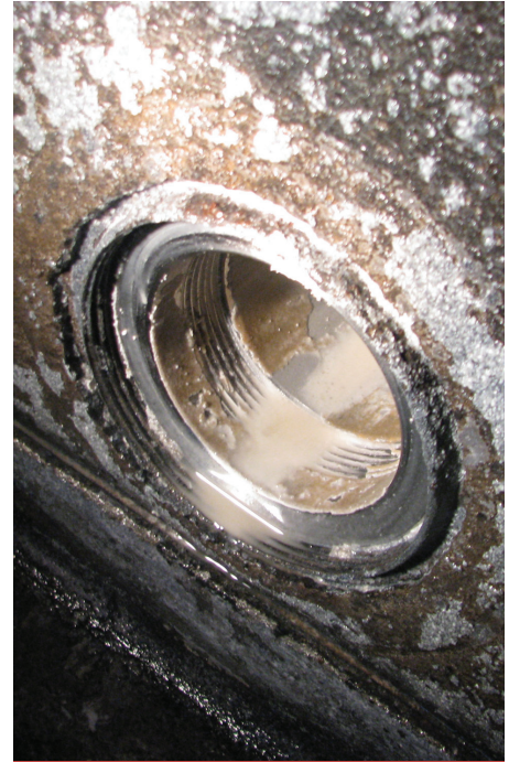
A view from inside a 3 inch valve. Note the distance from the floor of the tank.
