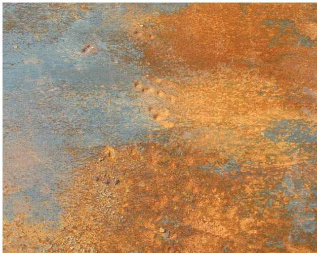
If a tank just has surface pitting (pits that aren't too deep), a good coat of paint can generally allow you to get a lot more service from the tank.
