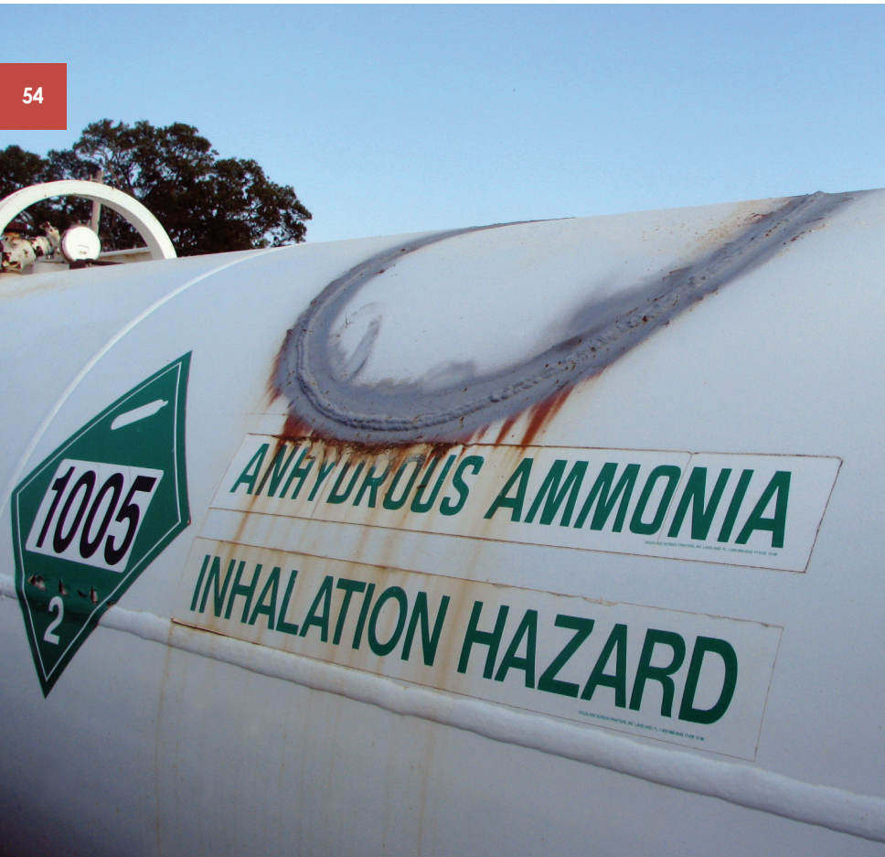
An access hole was cut into this tank to repair the internal baffles. This process is acceptable as long as the repair shop has the proper credentials and follows the correct procedures.
