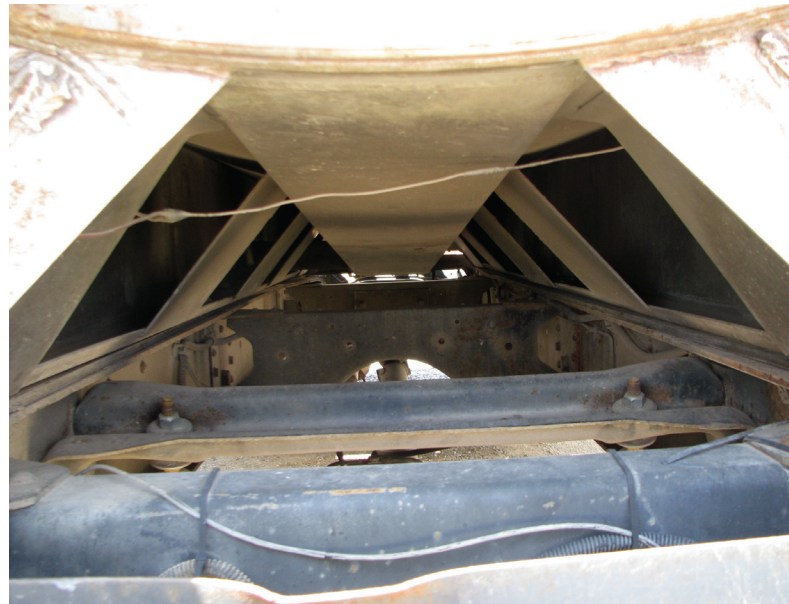
This view from the rear of the tank shows the gradual slope of the trough toward the front.
