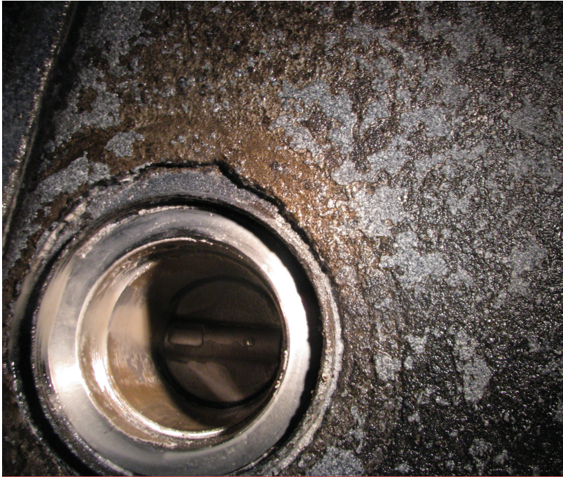
This photo shows the space between a stainless steel fitting and a mild steel tank. The space should be welded with a 309 grade welding rod to prevent product from getting between the tank shell and the fitting.
