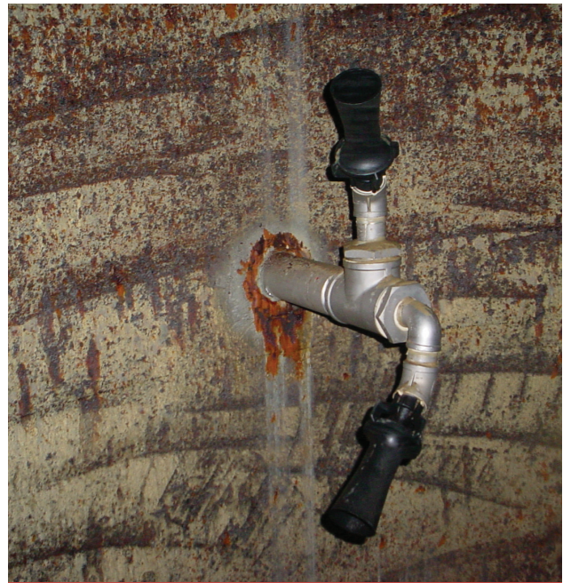
This device agitates the contents of a tank to help prevent buildup of salts and other deposits.
