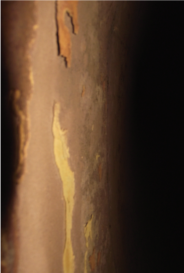
The sidewall of this tank shows significant corrosion. The outside might look clean, but it would not be a good idea to purchase this used tank. Be wary — a fresh coat of paint can be hiding a rusted or unclean steel surface that will not function long.
