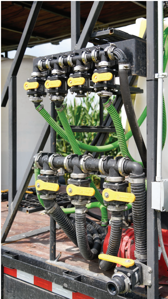
The more the pump is asked to do, the more the flow of the fluid to its final destination is reduced.
