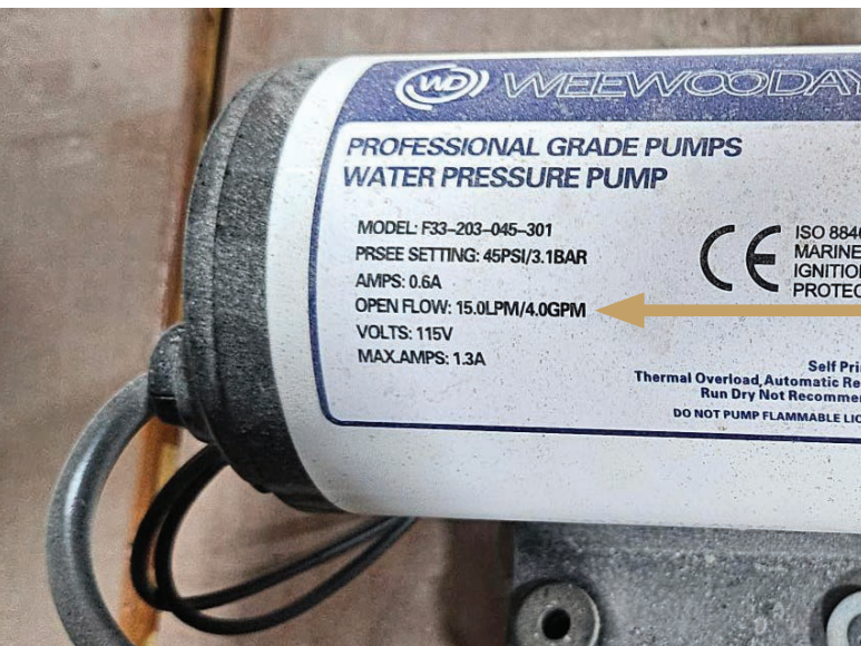
This pump moves 4 gallons per minute and is dedicated to moving fresh water to the batch tank.
