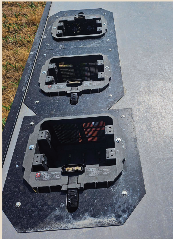
Coolers and the battery chargers are located at the top and side edge of the platform.
