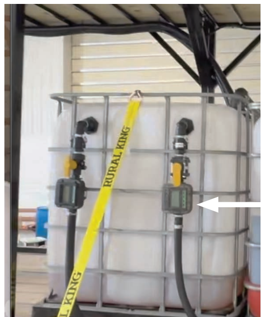
Metering chemical with a flowmeter when going from a larger chemical tank into the mixing tank.
