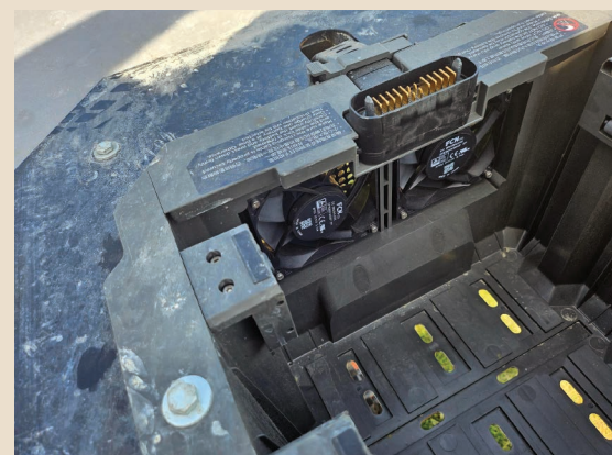
A close-up view of the fans within the cooler used to cool batteries. However, the batteries are not protected from sunlight while charging.
