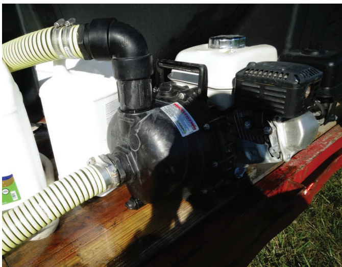
A pump showing its inlet to allow fluid to enter and an outlet to move the fluid forward to its desired destination. In this example, suction hoses are used to pull in and push out the liquid.
