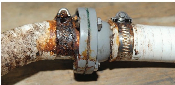
Examples of corroded standard clamps and T-bolt clamps from weather and chemicals.
