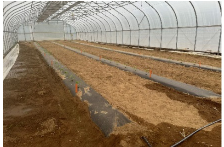
Figure 17. Rainwater seeping into a high tunnel from the sides.
