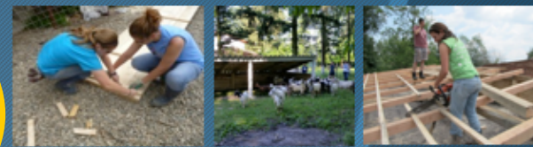
Examples of various construction projects. (Left to Right) Building the frame for new footer. New lean-to goat shelter. New roof on swine facility.
