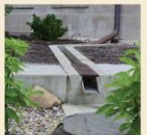
Concrete channels & drain grate
