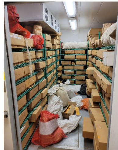
Figure 10.5 Typical cold room
